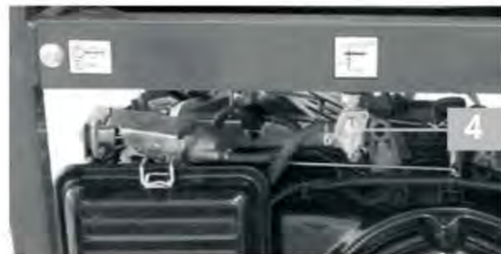
Fuel valve (OFF)
